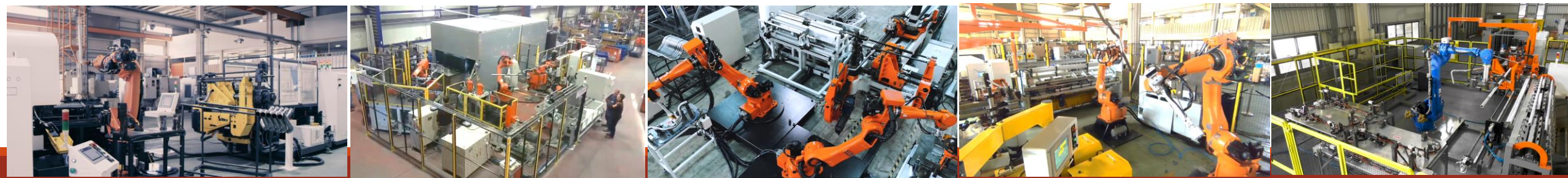
Automation work cell
